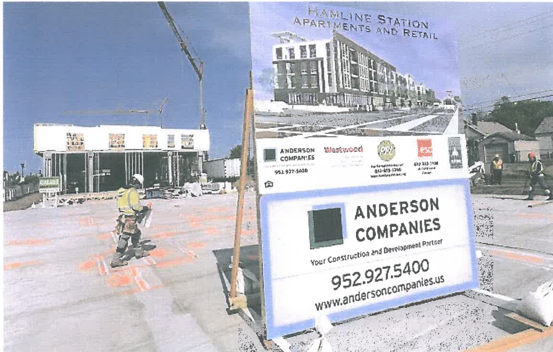
In this pre-construction picture, work had yet to be completed at Hamline Station on the former Midway Chevrolet used car lot at 1333 W. University Avenue, pictured in May 2015. Project for Pride in Living redeveloped the site into a $28 million, two-building, block-length affordable housing development with 108 apartments. (Pioneer Press: Jean Pieri)
